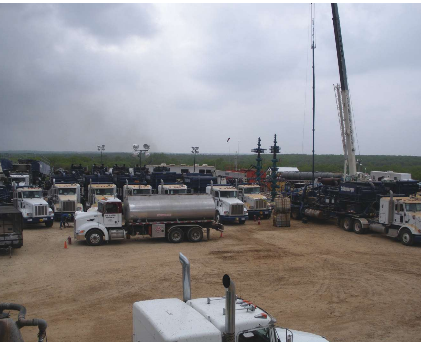
Two wells are completed simultaneously with a zipper frack in La Salle County, Texas. (Image courtesy of ZaZa Energy)
