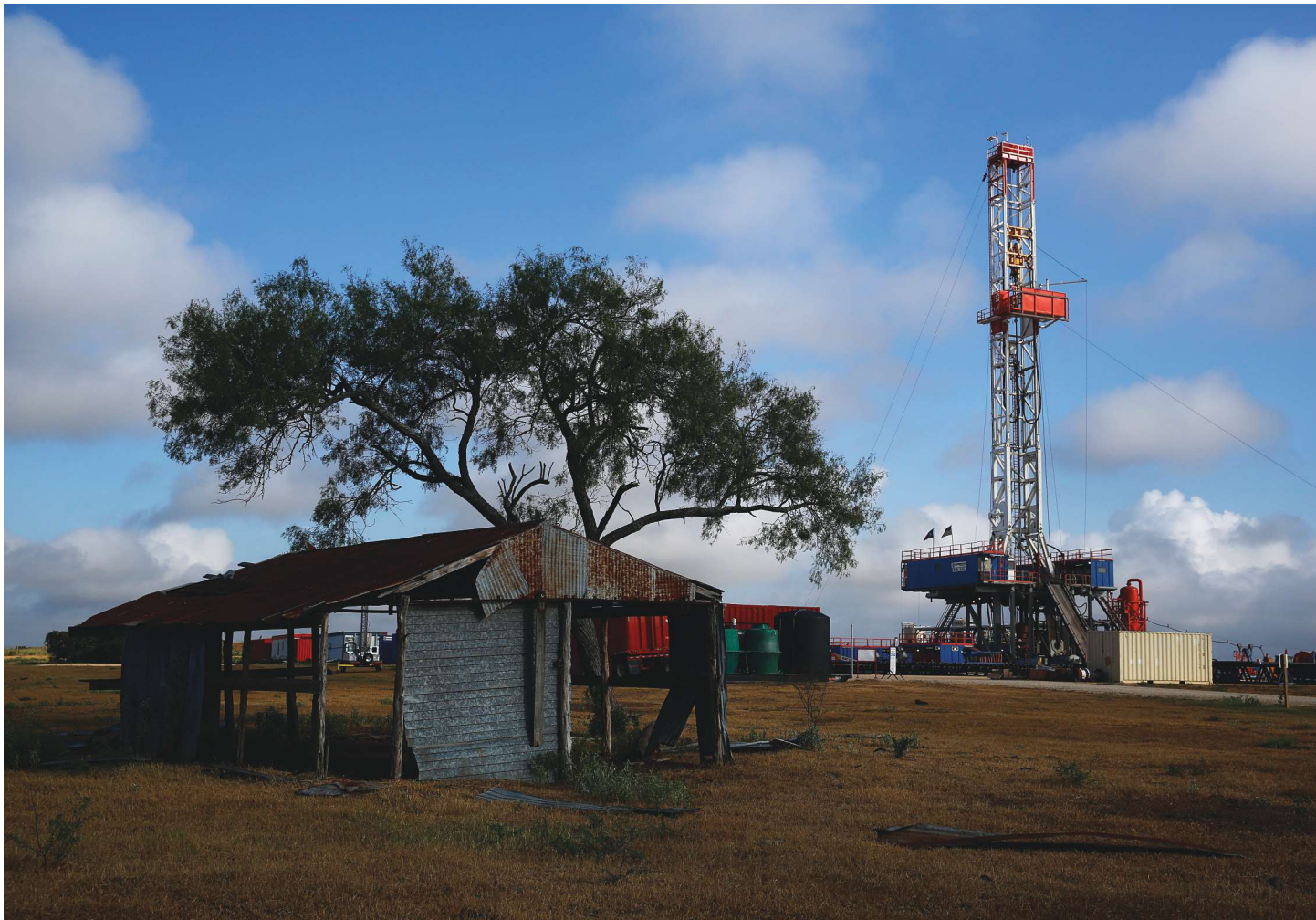
Patterson UTI Energy's Rig 246 drills ahead on the Riedesel 01-02H pad site for Pioneer Natural Resources Co. in the Eagle Ford Shale play near Yorktown, Texas. (Photo by Tom Fox, courtesy of Oil and Gas Investor)
