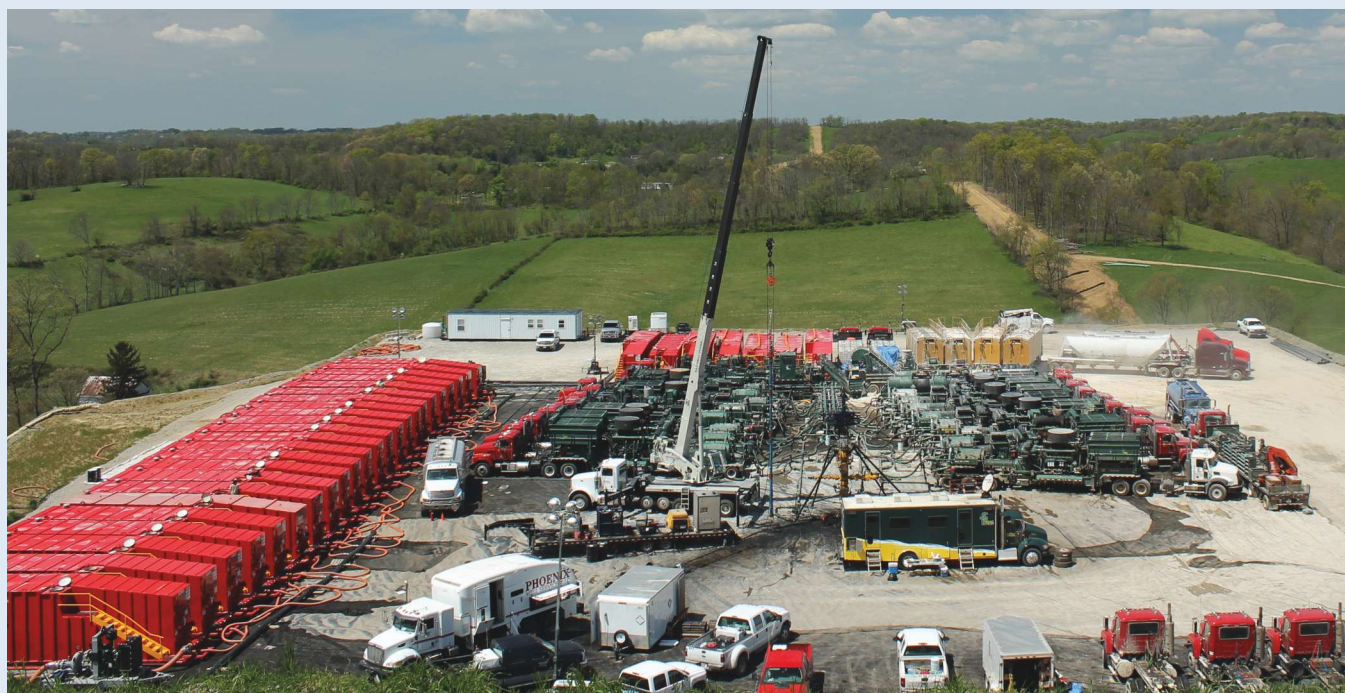
A frack job is underway on a Rice Energy well in Pennsylvania. (Photo courtesy of Rice Energy)
