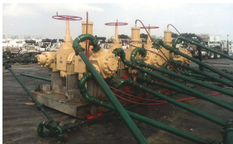
This Cameron Generation I frack manifold (an arrangement of flow fittings and valves installed downstream of the frack pump output header and upstream of each frack tree served by it) used in the Marcellus is an integrated skid design for up to 7 1 / 16 -in. 15,000-psi operations. (Photos courtesy of Cameron)
