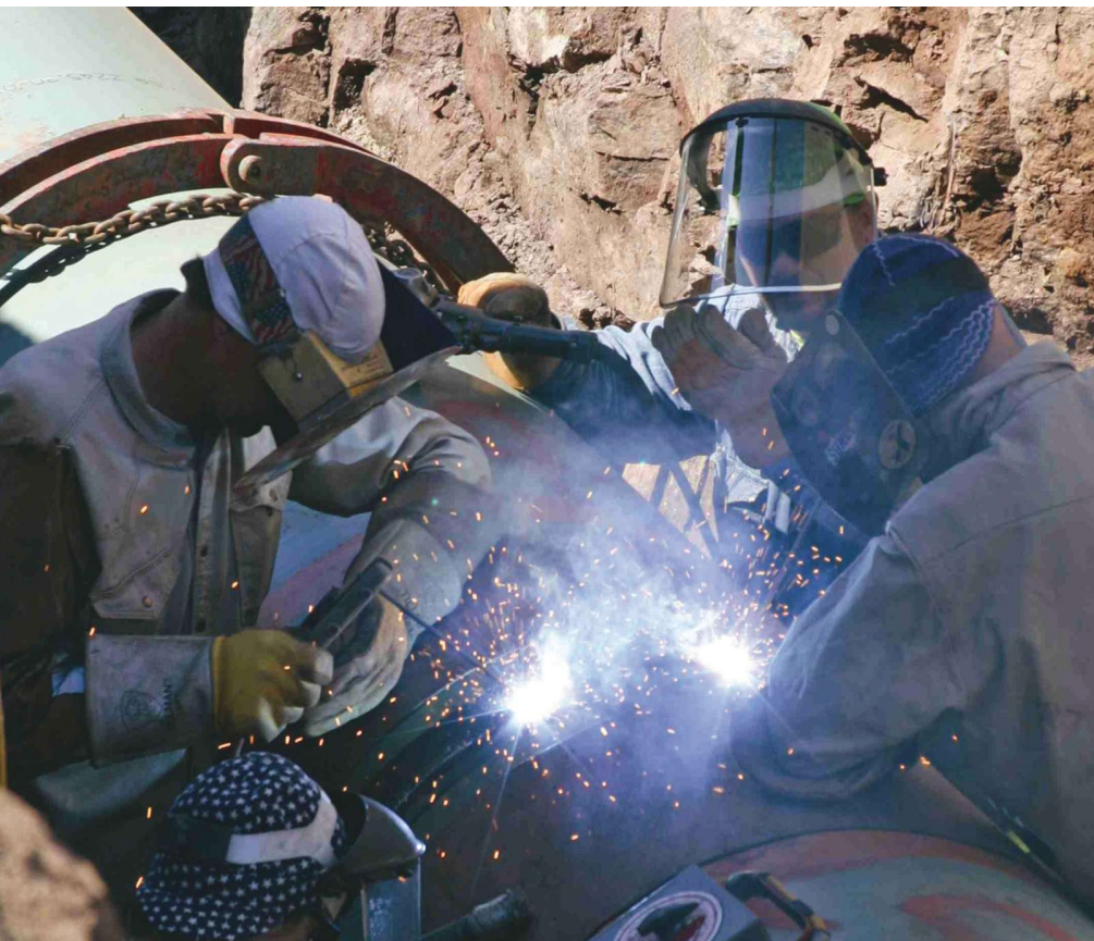
Spectra Energy is among several operators helping to open up the Northeast markets for Marcellus and Utica producers through the construction of several pipeline expansions, including its TEAM 2014, AIM and Atlantic Bridge projects. The company’s Algonquin Pipeline is one of two systems that currently move Appalachian volumes into New England. (Photo courtesy of Spectra Energy Corp.)
